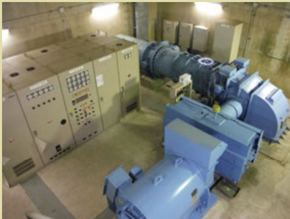
Hydroelectric power generator
